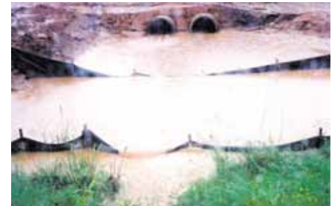
Makeshift "dams" to slow road project runoff help reduce erosion, but are rarely adequate. Not only does the sediment pollute receiving waters, the soil lost must be replaced at great expense. Photo by Rick Bryan.
