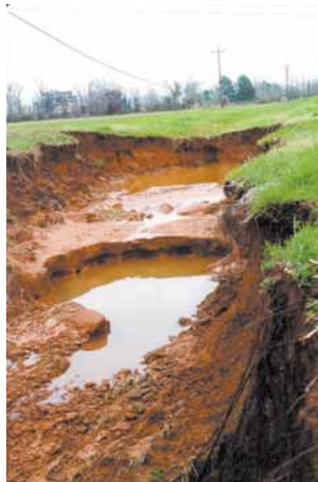
Gully washed along inadequately protected road bank. Photo by Rick Bryan.
