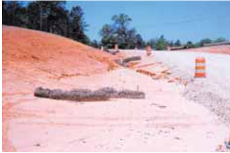
Road construction is a significant source of non-point pollution that is challenging to control, particularly under Louisiana's typical torrential rainfalls. Photo by Rick Bryan
